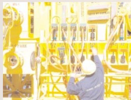
Taken during site integration testing, this Ocean Design, Inc. technician checks the hybrid connectors installed on a King's Peak subsea junction box (KOP).
